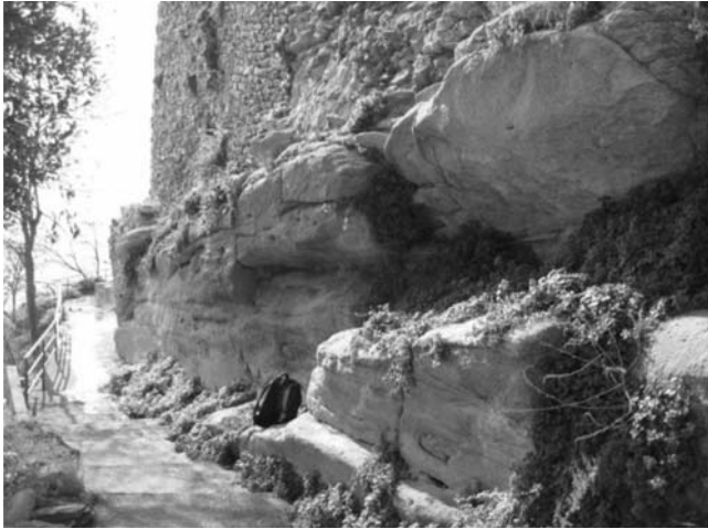
Fig. 8: Part P13. Underexcavated slope along a fault scarp. The wall was founded close to the edge. The toppling or the rupturing of the rock mass could cause extensive damages to the monument.
