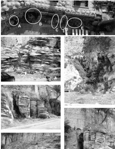
Fig. 5: Part P5. View of the slopes below Imaret monument intersected by the faults presented in the map of Fig. 1. The deterioration of the rock mass along the major tectonic lines cause serious rock slope stability problems threatening the monument. The letters pointing the various unstable locations correspond to the homonymous pictures (5A to 5E).
