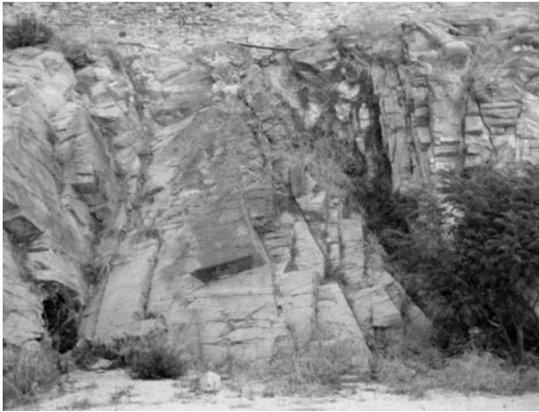
Fig. 4: Location P2. An oversized rock wedge that probably failed during the excavation of the small tunnel appearing at the base of the slope, on the left side of the picture. The extension of the failure could very easily damage the Byzantine wall.
