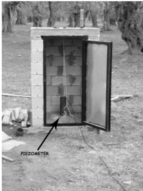
Fig. 5: In Area C (Thassos island), STATION 4 was plunged in the piezometer of an existing borehole and a small lodge to protect the sensors was constructed.
