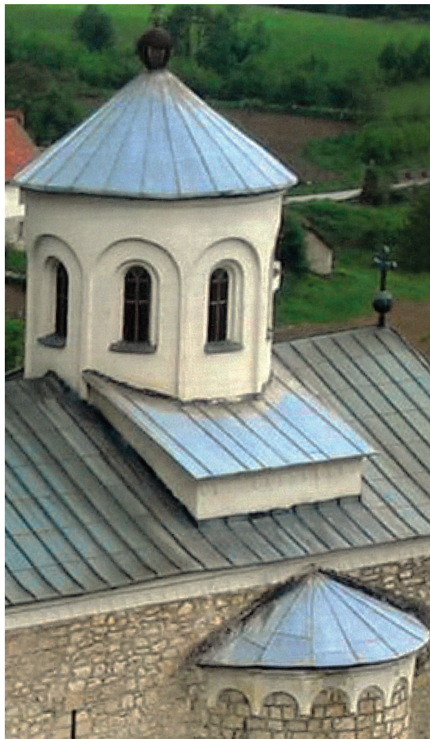
Fig. 6. Bosnia, monastery of Paprača, church of the Annunciation. View of the dome and the south niche after conservation works.
