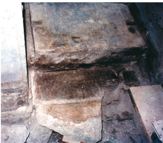
Fig. 6. Panagia Skripou. Narthex, south door. (a) The remaining timber tie-beam and the frescoes covering the walls. (b) The threshold of the south door with parts of the original marble floor.
