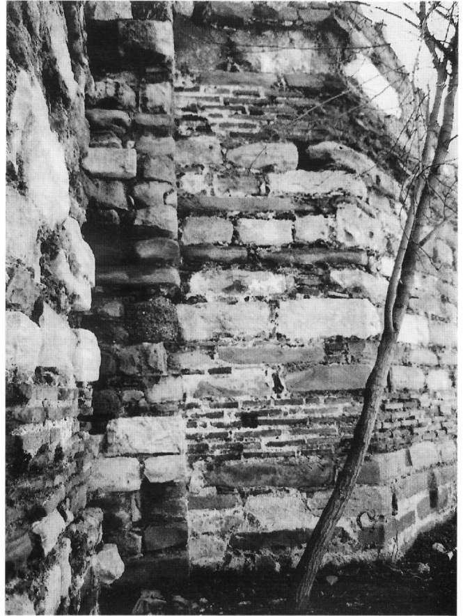
Fig. 10. The brick courses end at the corner where walls 'e' and 'd' of tower II meet.
