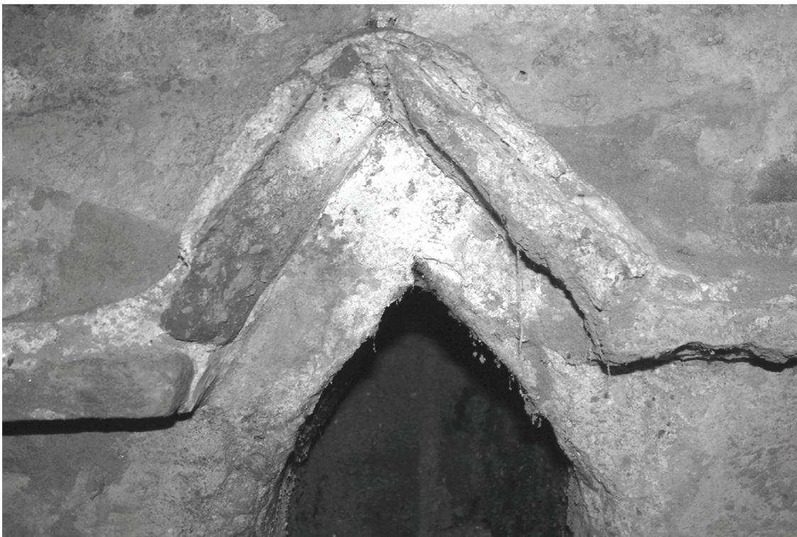
Fig. 19 The arched spring with the band of red tiles and the layer of plaster over it.
