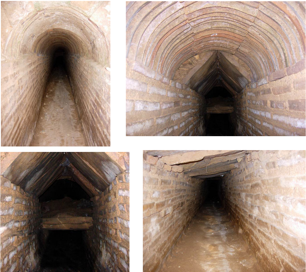
Fig. 3. The inclined gallery of the Hadrianic aqueduct at the Olympic Village; various types of support with standardized bricks are shown (Horne, 2009).
