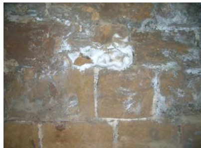
Figure 2 - Salt efflorescence on the external wall of Koule Castle, Heraklion, Crete.
