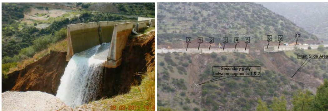
Figure 2 - Canal segment failure (left), Main slide shortly after occurrence (right).
