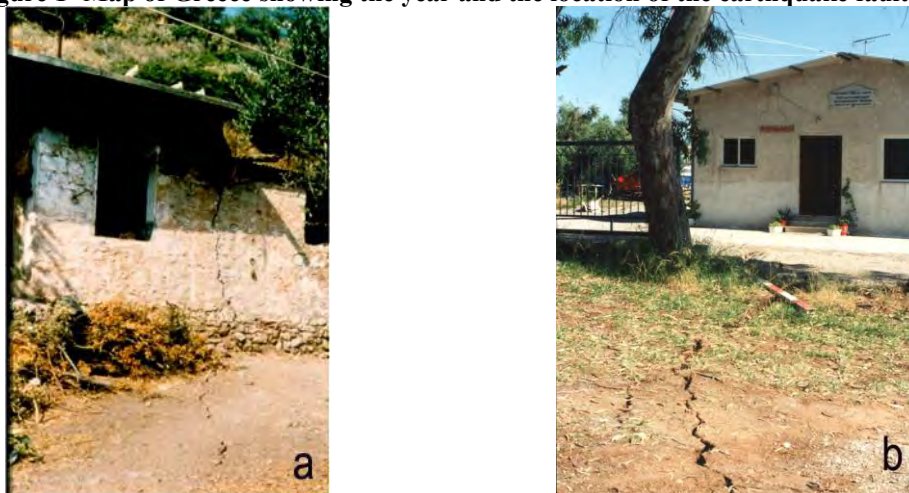
Figure 2- Open seismic cracks, without vertical displacement, formed during the 1986 Kalamata (a) and 1995 Aigio (b) earthquakes.
