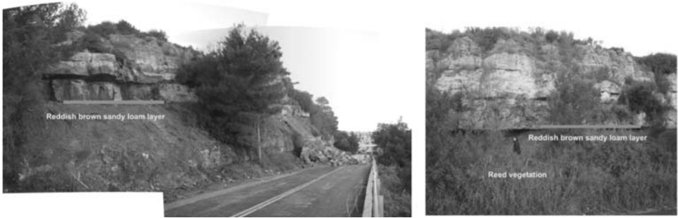
Fig. 7. The layer of reddish-brown sandy loam is slowly washed out by the percolating water from the overlying limestone (note the beginning of undercutting). The water favors thick reed vegetation. It is a matter of time this slow process to undercut the limestone causing a rockfall in this place in the future.
