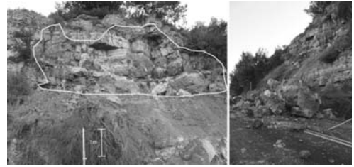
Fig. 4: Source area of the December 21, 2009 rock falls.
