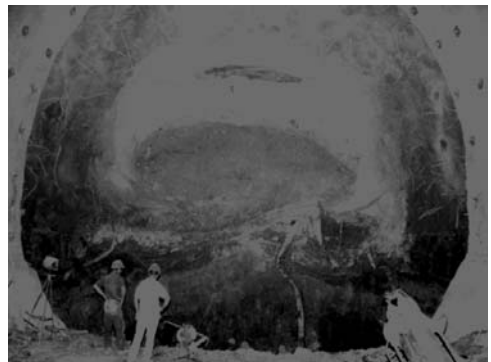
Fig. 7: Old collapsed tunnel during re-excavation.
