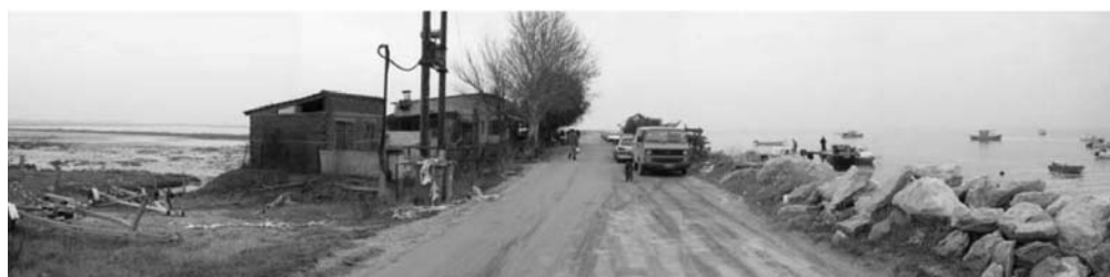
Fig. 4: View of the main embankment constructed in the South of Kalochori. On the right side of the embankment the sea level is about 0.5m below the road level. On the left (interior) side, the lagoon water level is 4 to 5m below the road level. Concluding, the inland is at least 4m below the sea level.
