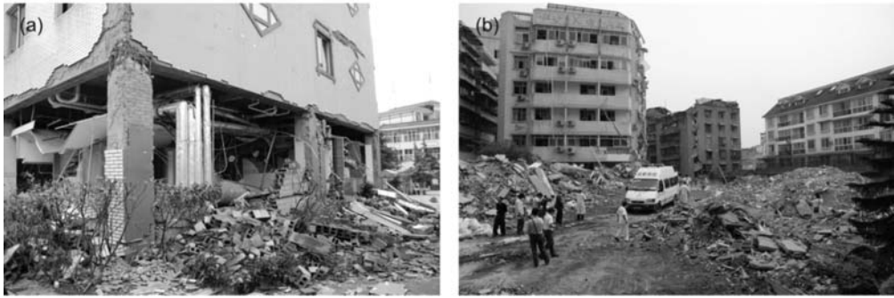
Fig. 3: View of a recently constructed building at the suburbs of Dujiangyan (Guanxian) with serious structural damages on the ground floor props. (type of construction D, damage degree 4) (a) and view of a hospital unit in the same town that totally collapsed (type of construction D, damage degree 5) (b).
