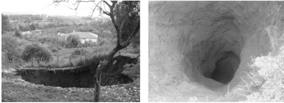
Fig. 7: The sinkhole in Temploni are.
