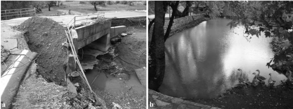
Fig. 2: (a): Disasters caused to Giannoulis Stream, upstream Logaras Spring by the storms of November 2007. (b): The lake formed at Logaras Spring, with muddy water after storms and the subsequent floods of November 2007.
