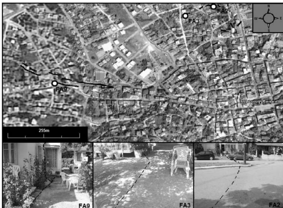
Fig. 4: Satellite pictures (from Google Earth) pointing the location of the surface raptures along Farsala town. Pictures FA2, FA3 and FA9 show roads and buildings damaged by the surface raptures.
