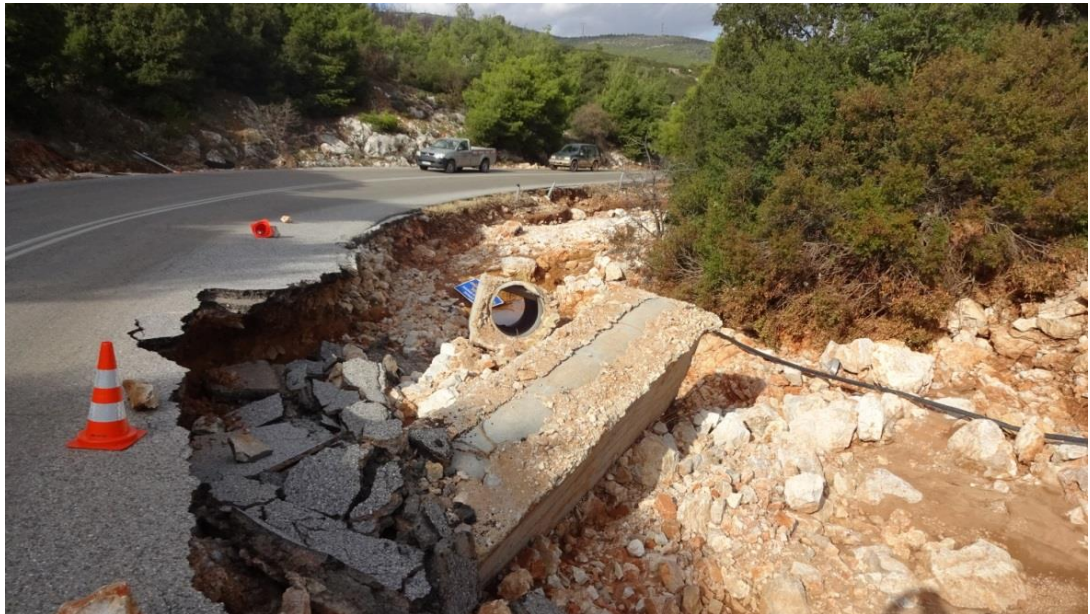
Fig. 6: Erosion of road 3 of Mandra-Thebes (E962) from the flood of 14-15 / 11/2017.
