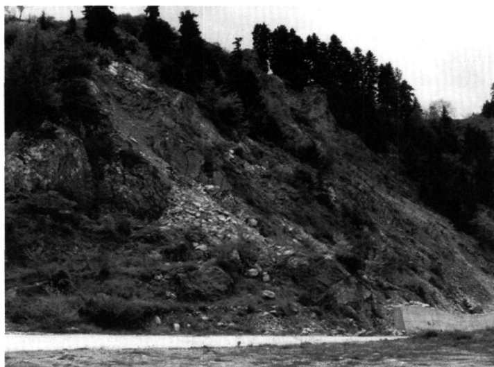
Figure 4 - Landslide No2 (cross-section BB')
