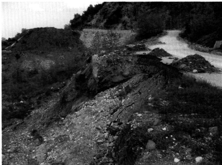
Figure 3 - Landslide No1 (cross-section AA')
