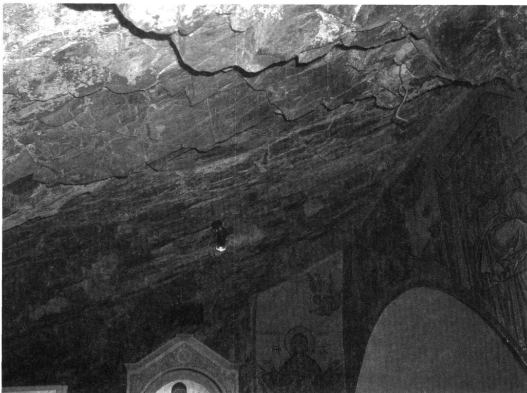
Figure 7 - Ceiling view of section B. Unsupported Section. The north western corner of the section, appearing the rock falls, is clearly presented
