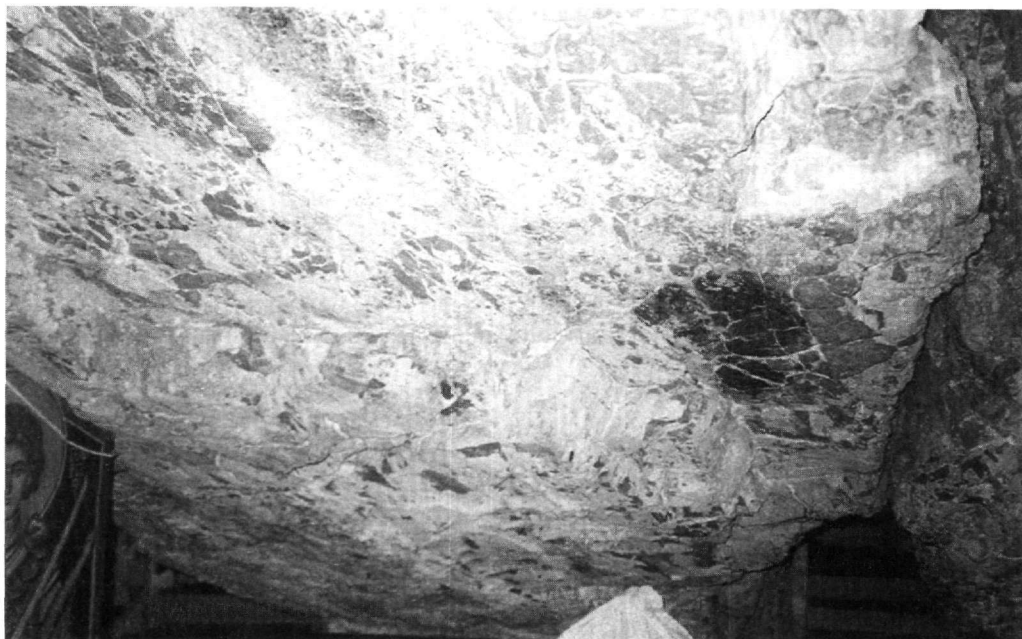
Figure 8 - View of the wedge formed by the faults intersecting the cave. The concrete column constructed for the support of the wedge is visible on the left side of the figure
