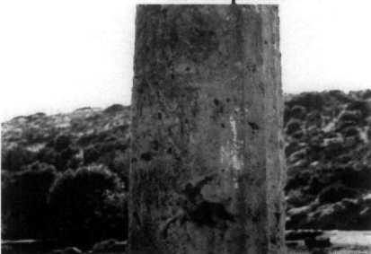
Figure 18 - Intence decay form on sandstone type III
