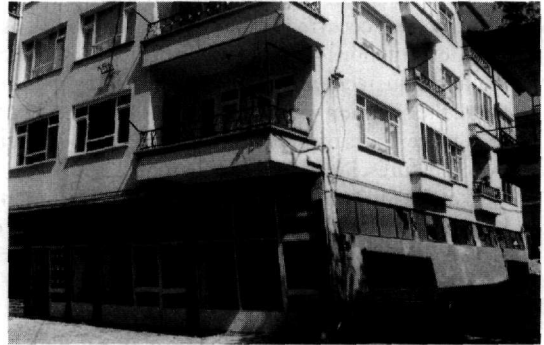
Fig. 6 Reinforced concrete frame structure in Yalova that displayed first story column-hinge deformation, but did not collapse (damage degree 4).
