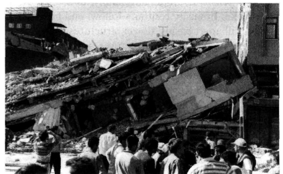
Fig. 4 Reinforced concrete frame structure that collapsed in Gölcök town (damage degree 5).
