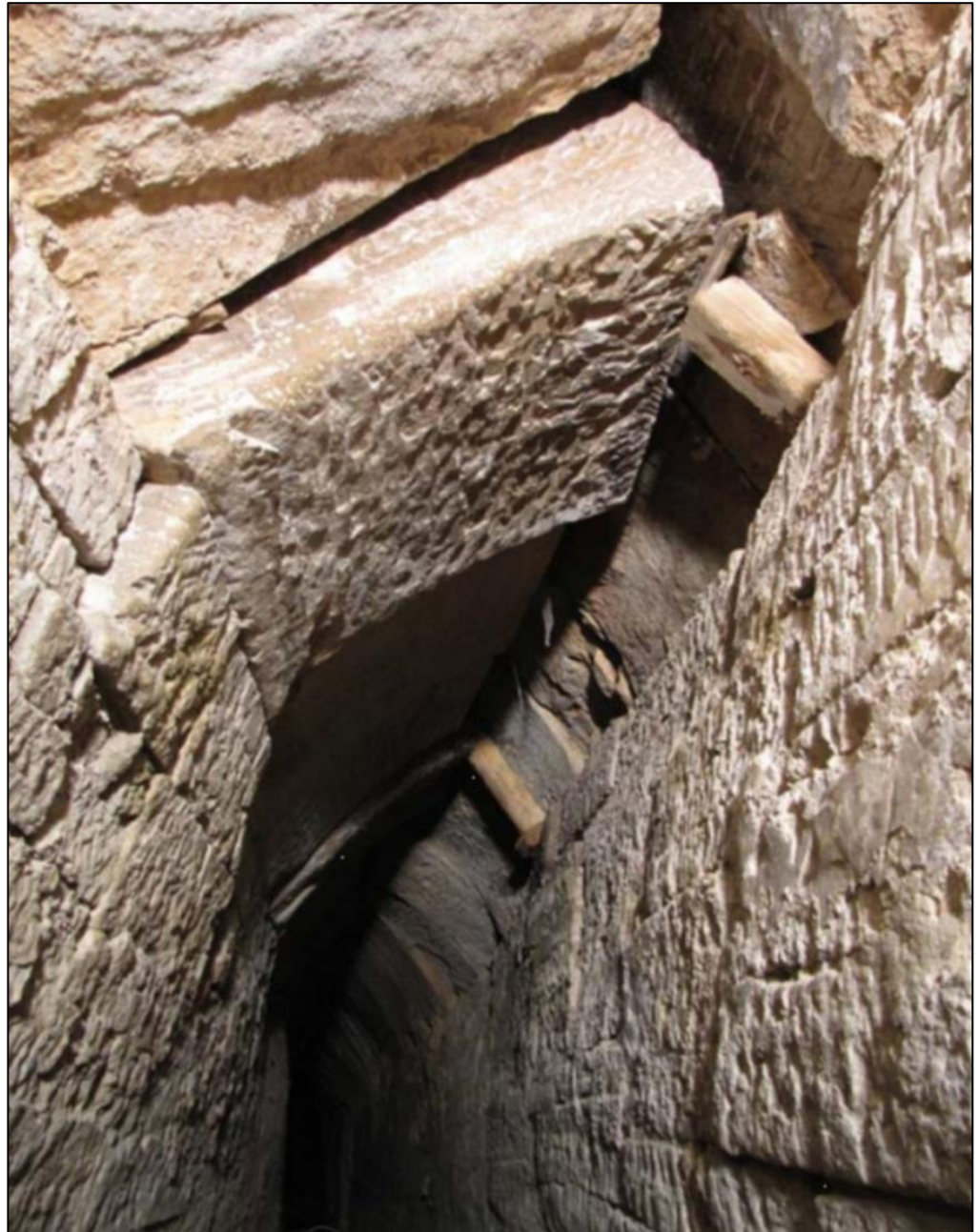
Fig. 13: The tunnel at ch. 0+130 with dislocated roof stones.
