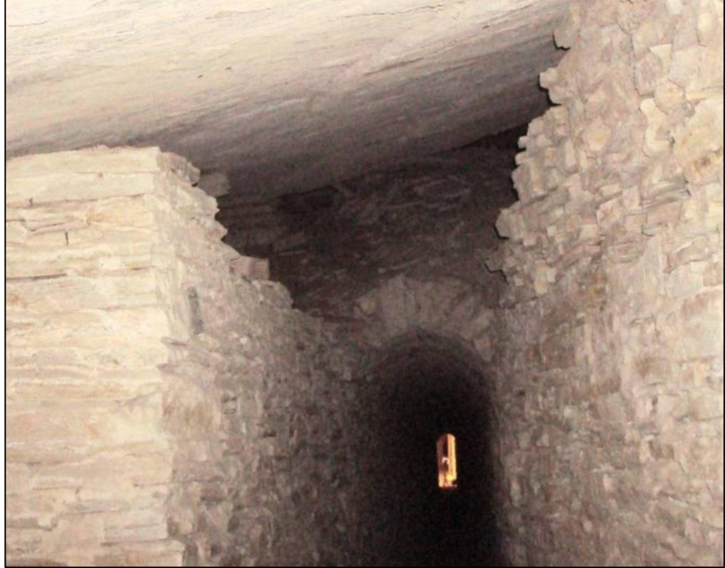
Fig. 17: Roman type wall of the north portal. The tunnel roof (geological bedding is subparallel to the tunnel axis) has collapsed on the arch of the wall. For a limited length the walls are vertical up to the tunnel roof.
