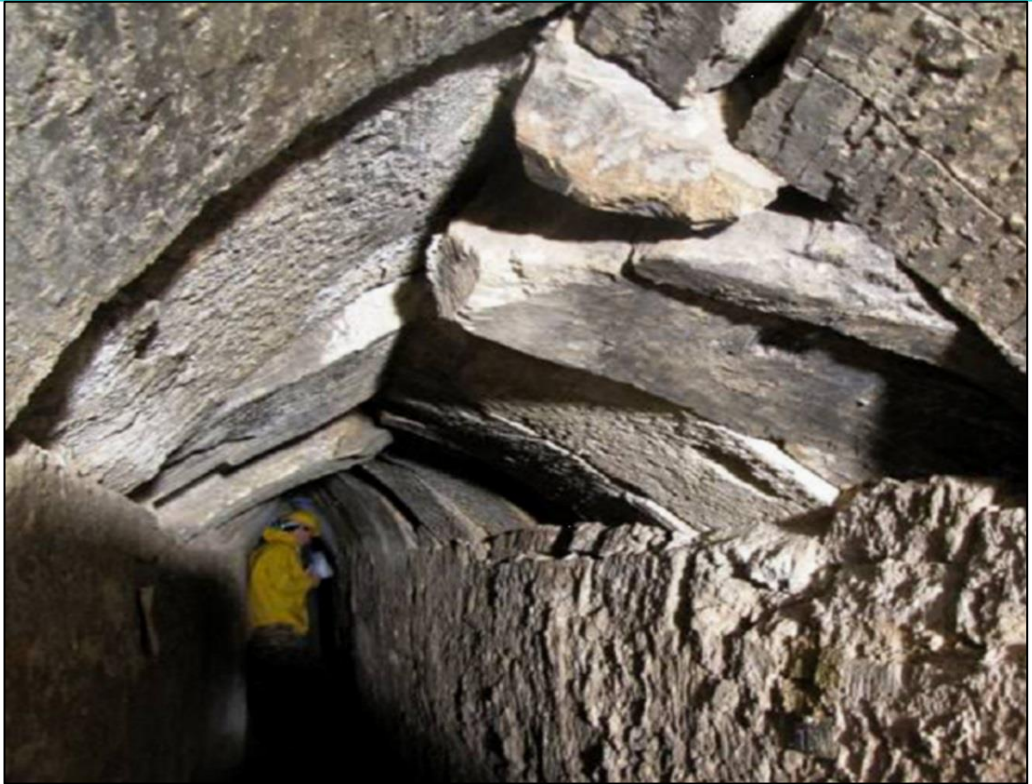
Fig. 20: Fractured and displaced arched stones at chainage 0+180.
