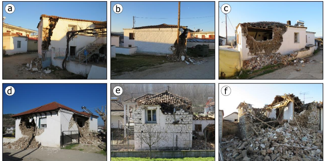
Fig. 7: (a, b) Vertical cracks and gaps were frequently formed and propagated along the height of the bearing wall intersections. This damage is attributed to the absence of horizontal banding means, which could provide structural integrity. Examples from Mesochori village. (c, d) Failures of the upper part of the walls were also attributed to the interaction of roof structure and perimeter walls. Examples from Mesochori (c) and Damassi (d) villages. (e, f) Damage were also attributed to poor mortar and poor workmanship resulting in partial or total collapse. Views from Mesochori village.
