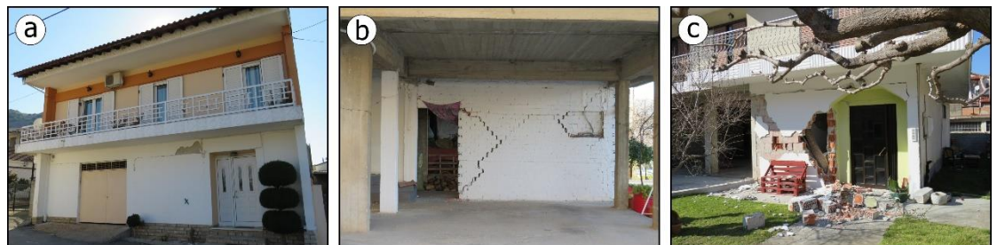
Fig. 9. Few earthquake-affected reinforced concrete buildings suffered non-structural damage varying from slight detachment of the infill walls from the surrounding reinforced concrete frame (a) and cracking in the infill walls (b) to partial collapse of the infill walls (c).
