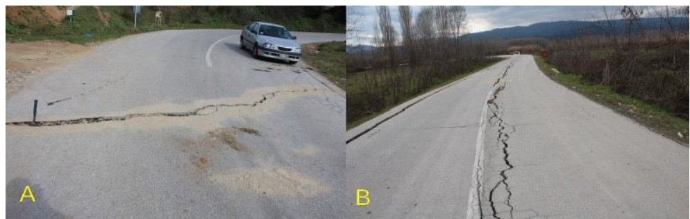
Fig. 16: Secondary cracks due to lateral spreading and associated liquefaction NW of Mesochori village.
