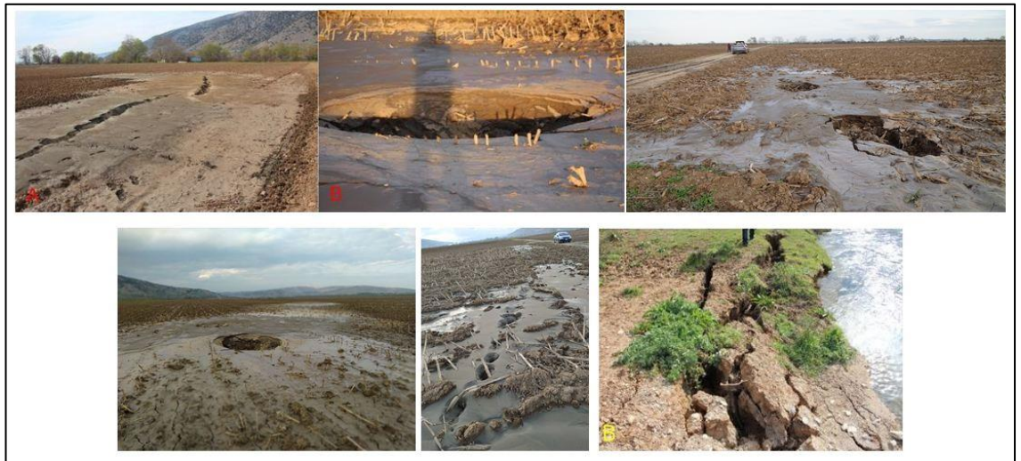
Fig. 12: Examples of sand flows, sand boils and lateral spreading in the liquefied area SE of Pineiada village.
