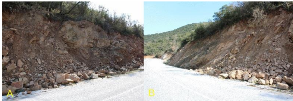
Fig. 15: Rock falls and slope failures along the country road to Vlachogianni village.
