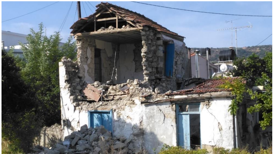
Fig. 2: Structural damage in a traditional house during the 2021 Arkalochori earthquake (after ITSAK, 2021), estimated to represent a model for the damage implied by Limbritis. The only exception is the rooftiles which derive from a later renovation; Originally the roof was made of wood and earthen material. This type of damage in weak walls could be easily repaired shortly after an earthquake.
