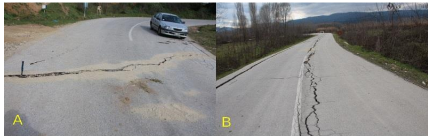
Fig. 16: Secondary cracks due to lateral spreading and associated liquefaction NW of Mesochori village.
