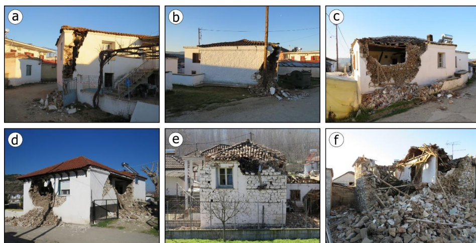
Fig. 7: (a, b) Vertical cracks and gaps were frequently formed and propagated along the height of the bearing wall intersections. This damage is attributed to the absence of horizontal banding means, which could provide structural integrity. Examples from Mesochori village. (c, d) Failures of the upper part of the walls were also attributed to the interaction of roof structure and perimeter walls. Examples from Mesochori (c) and Damassi (d) villages. (e, f) Damage were also attributed to poor mortar and poor workmanship resulting in partial or total collapse. Views from Mesochori village.
