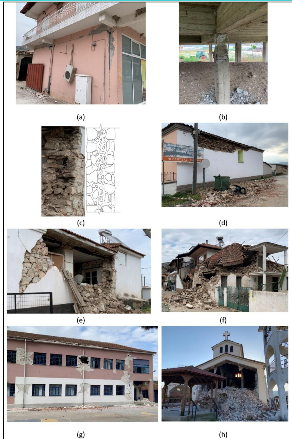
Fig. 13: a) Detachment of infill wall from RC frame in Damasi; b) Lack of proper detailing in an open ground floor in Damasi; c) Cross-section of a typical multi-leaf wall; d) Delamination of the outer leaf of the wall in a domestic building in Damasi; e) Out-of-plane collapse of masonry walls in Damasi; f) Out-of-plane collapse due to poor connection between the roof and masonry walls in Damasi; g) Damages in the School of Damasi; h) Out of plain failure of St Nickolas Church in Koutchochero.
