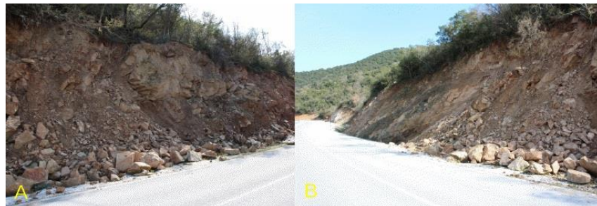
Fig. 15: Rock falls and slope failures along the country road to Vlachogianni village.
