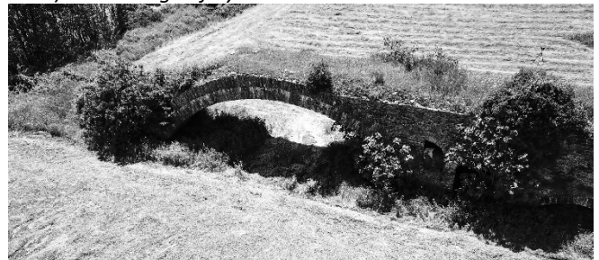
Fig. 8. The bridge of Kyra, current condition (photo of the authors).
