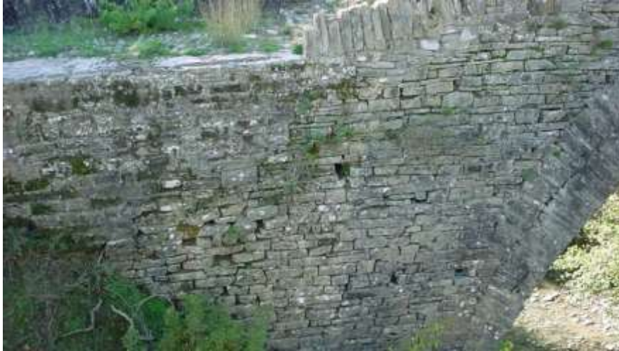
Fig. 2. Extensive loss of sandstone bonding mortar
