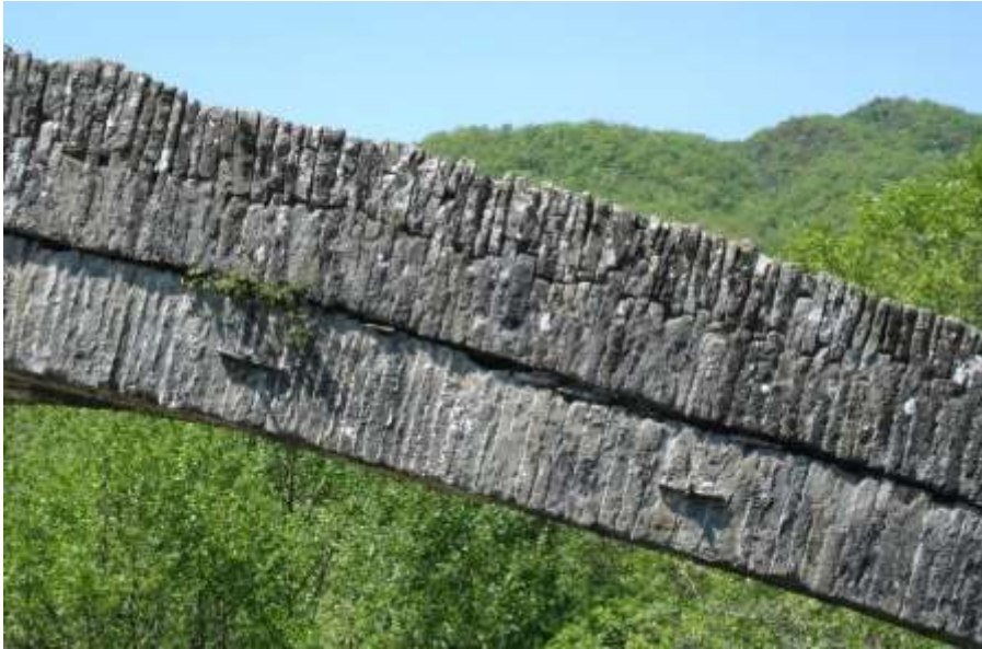
Fig. 4. Loss of contact between the two rings
