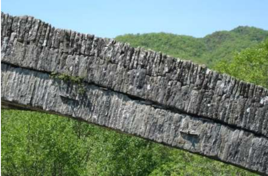
Fig. 4. Loss of contact between the two rings
