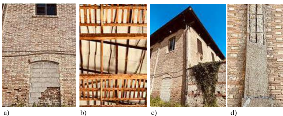
Fig. 11. Injuries on the case study: a) Crushing of masonry walls, b) Poor connection between adjacent walls, c) Decay of wooden beams, d) Detachment of the cover concrete from the pillars
