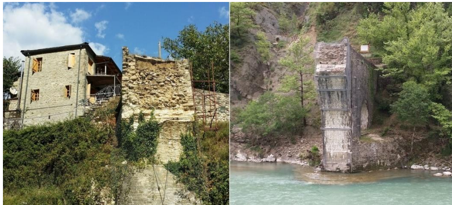
Fig. 6. Surviving sections of Plaka Bridge, September 2018. Left: part of east abutment and the Customs building. Right: West abutment and piers body.
