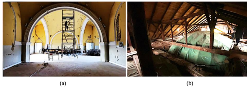
Fig. 4. The first floor (view towards West) damaged by the December 2020 earthquake (a) and attic with upper surface of the main timber dome (view towards West) (b)
