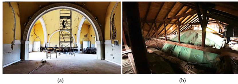
Fig. 4. The first floor (view towards West) damaged by the December 2020 earthquake (a) and attic with upper surface of the main timber dome (view towards West) (b)
