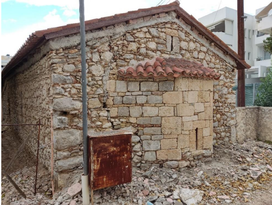
Fig. 3. South–East view of the church. Removal of plaster on the exterior masonry. (24/9/2022)
