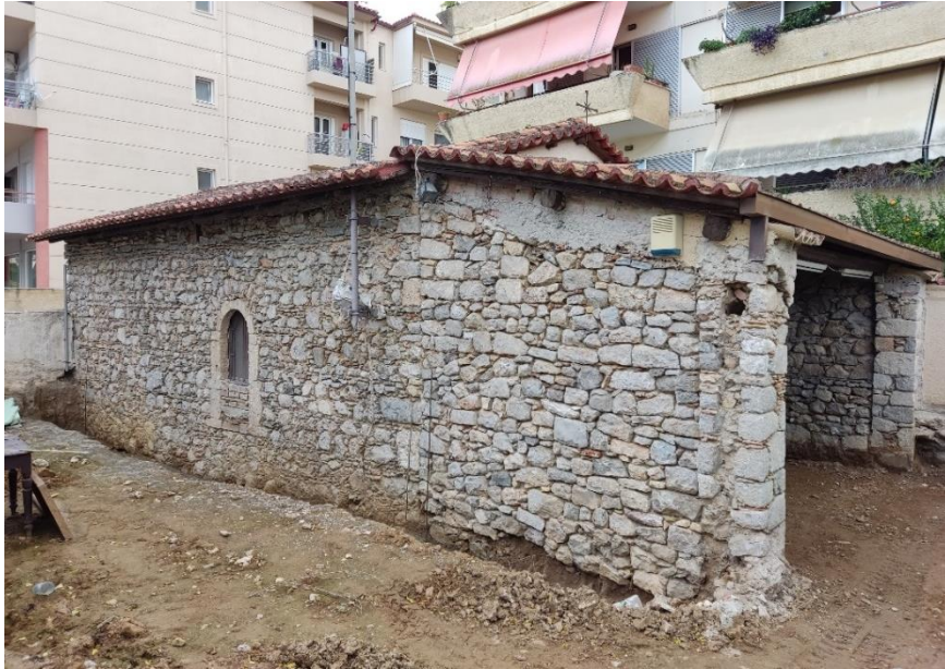
Fig. 2. North–West view of the church. Removal of plaster on the exterior masonry. Excavation of the northern part of the surrounding area. (24/9/2022)
