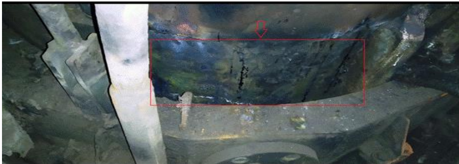
Fig. 15. Case study of melted casing steel due to overheating
