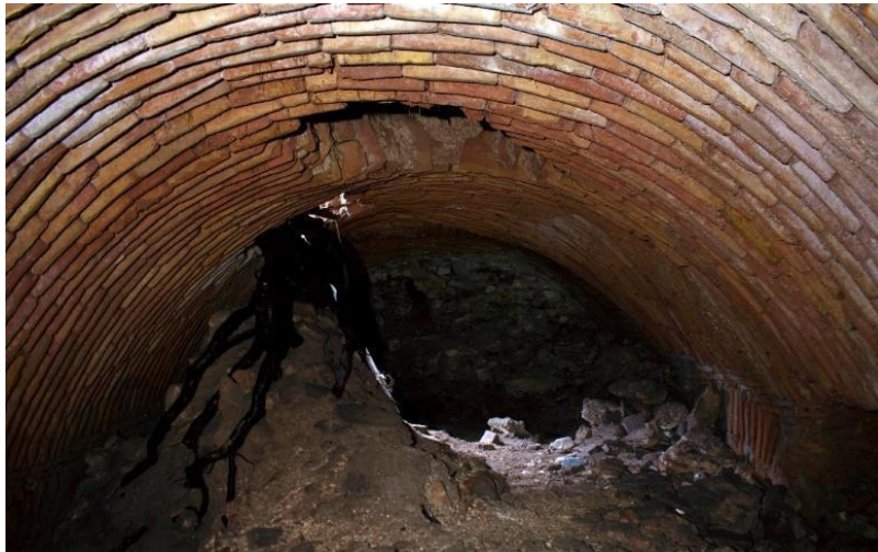
Fig. 14. View from the first vault under the northeastern wing of the Justinian's atrium.
