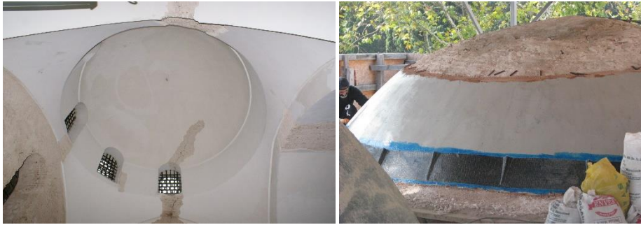
Fig. 26. View from the crack under the dome and CFRP intervention above the dome.
