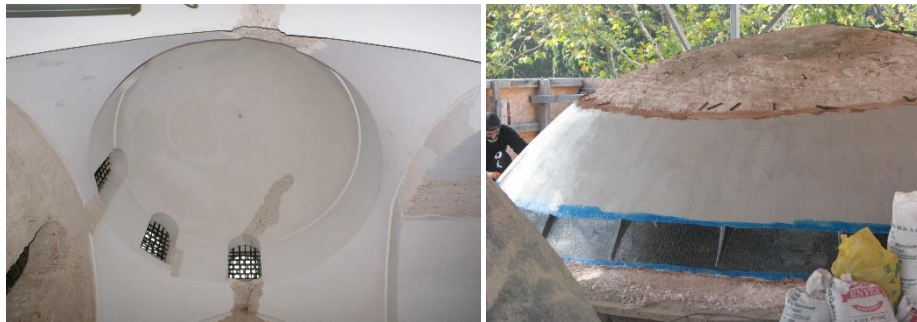
Fig. 26. View from the crack under the dome and CFRP intervention above the dome.
