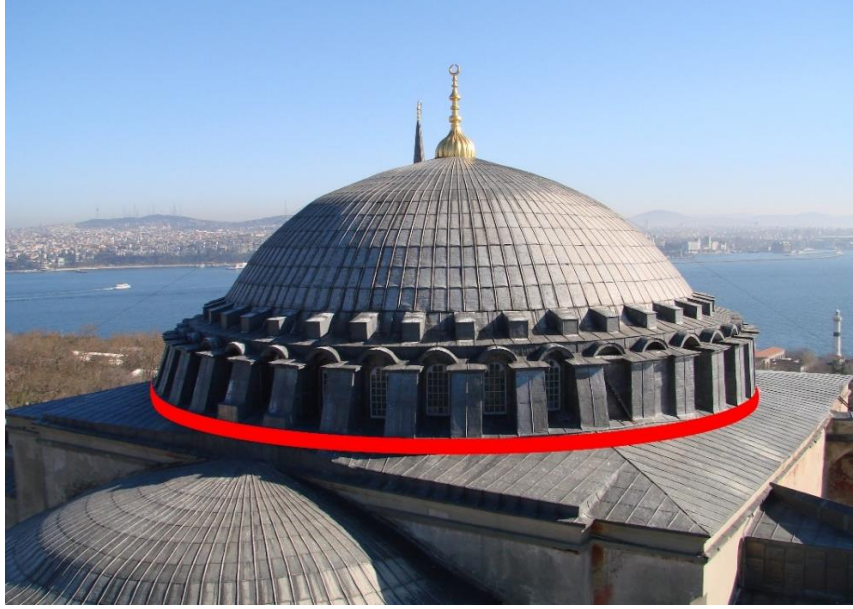
Fig. 17. Representation of the tension ring around the main dome of Hagia Sophia
