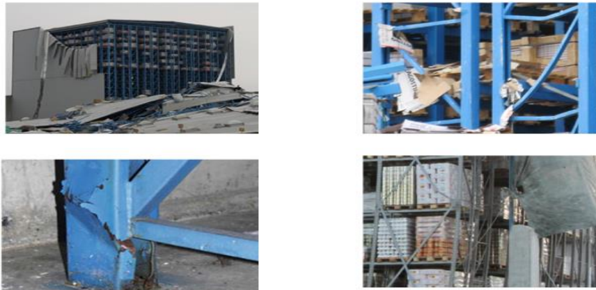
Fig. 10. Failure of steel racks making part, or not of the lateral load resisting system, Emilia earthquake, 2012 [70].
