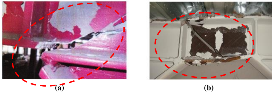
Fig. 8. Fracture of EBF's links, a) at hospital parking garage, b) at Pacific Residential Tower, [60].
