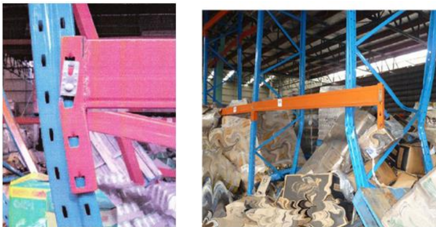
Fig. 9. Failures of steel rack pallets in Christchurch earthquake, 2011 [60].
