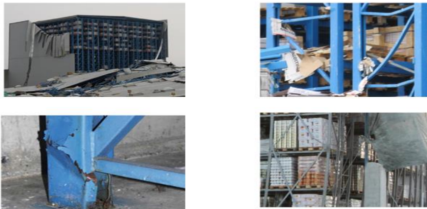
Fig. 10. Failure of steel racks making part, or not of the lateral load resisting system, Emilia earthquake, 2012 [70].
