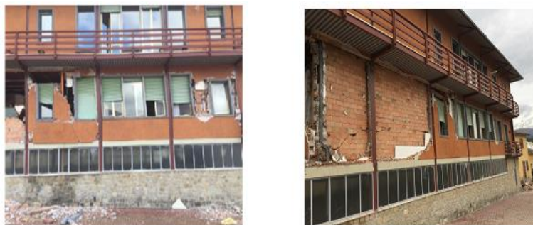
Fig. 11. Steel frame with infill masonry interaction, Amatrice earthquake, 2016, [74].
