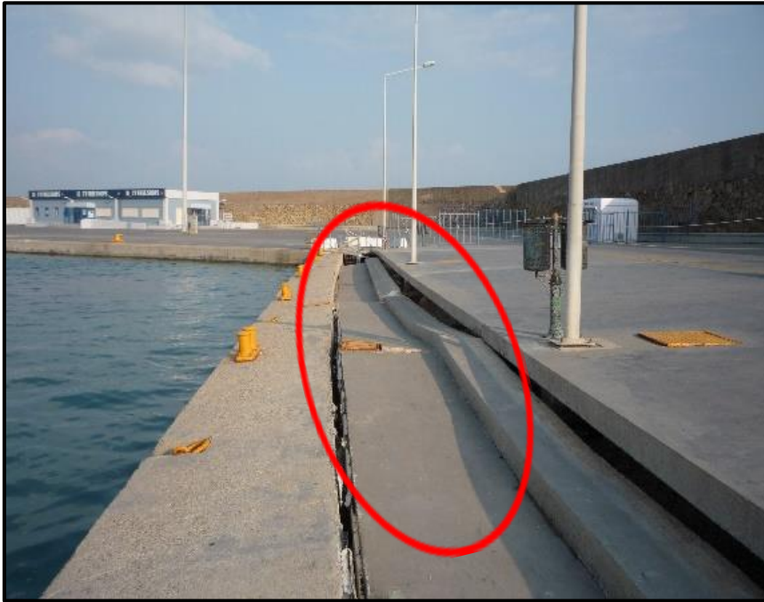
Fig. 5. Subsidence of sections of the commercial quay of Katakolo Port in 2009, circled in red. (Kiouisi et al., 2023)
