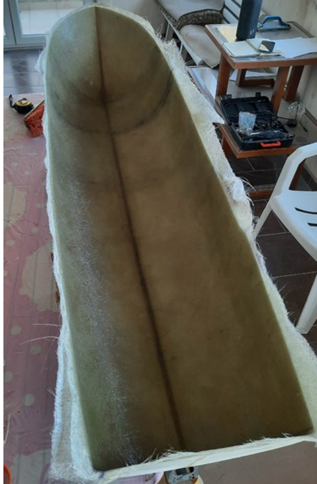
Fig. 29. Application of a final layer of polyester and fibreglass on the inner surface of the hull model
