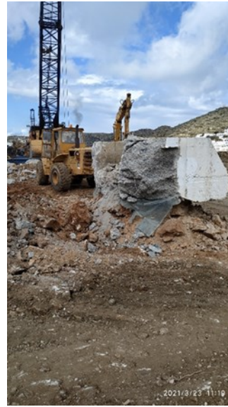
Photo 8. Several existed artificial blocks were damaged during transportation and used as embankment material
