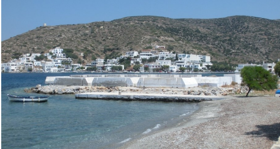
Photo 2. The new pier at Katapola beach on 2015, consisted of embankment material and three types of 17 concrete blocks, abandoned on site 10 years ago
