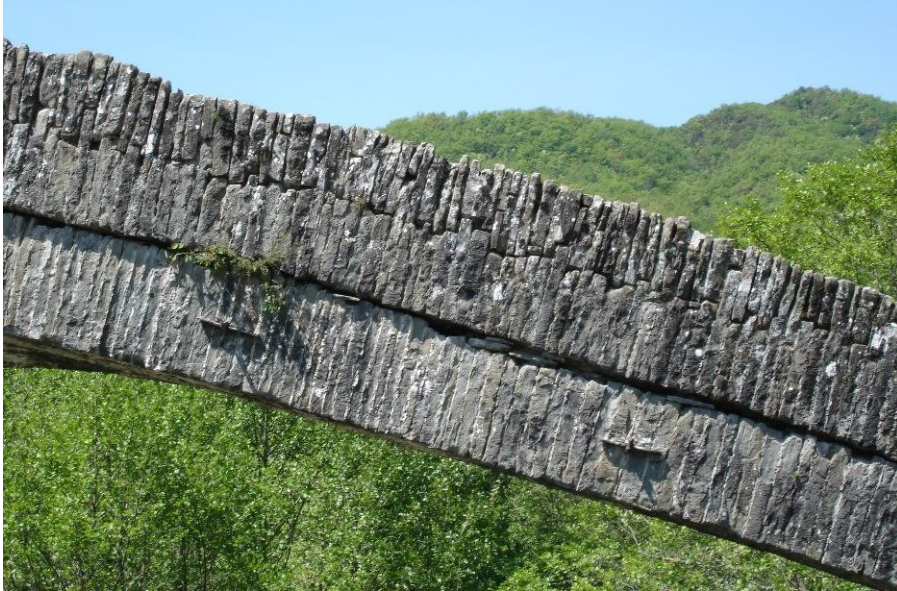
Fig. 4. Loss of contact between the two rings
