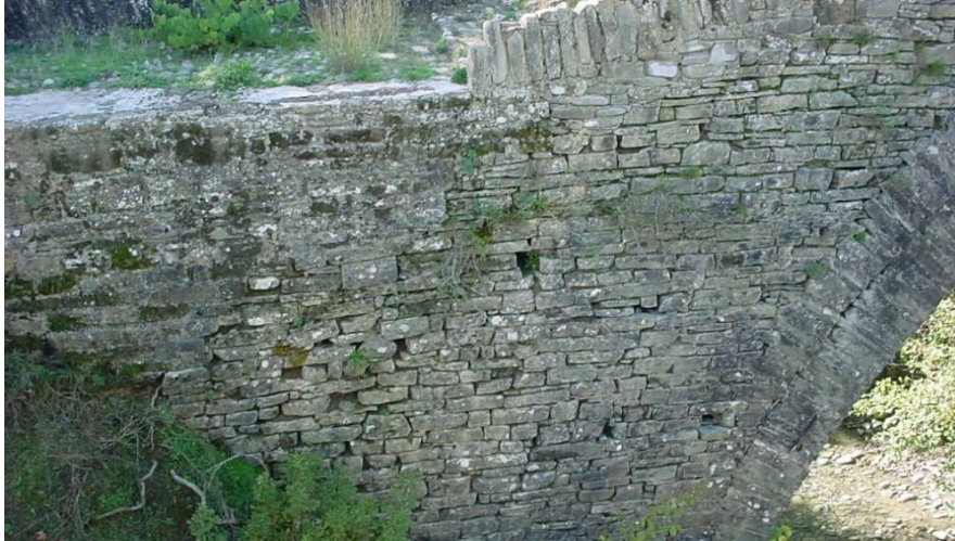
Fig. 2. Extensive loss of sandstone bonding mortar
