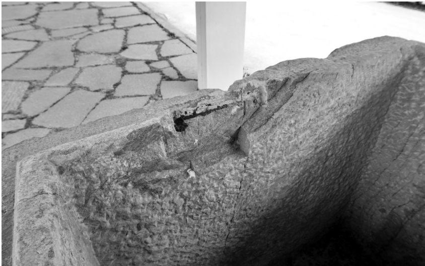
Fig. 5: Setting of a rusted iron clamp (photo by authors)
